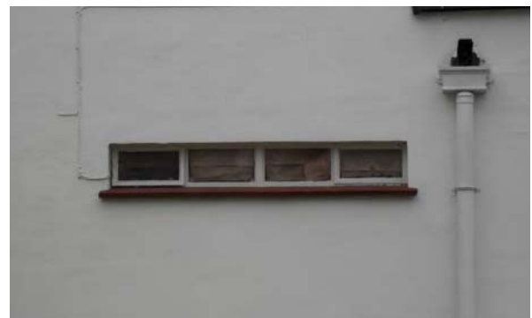
Picture 4.83 Flat window on number 5 Kerry Avenue
